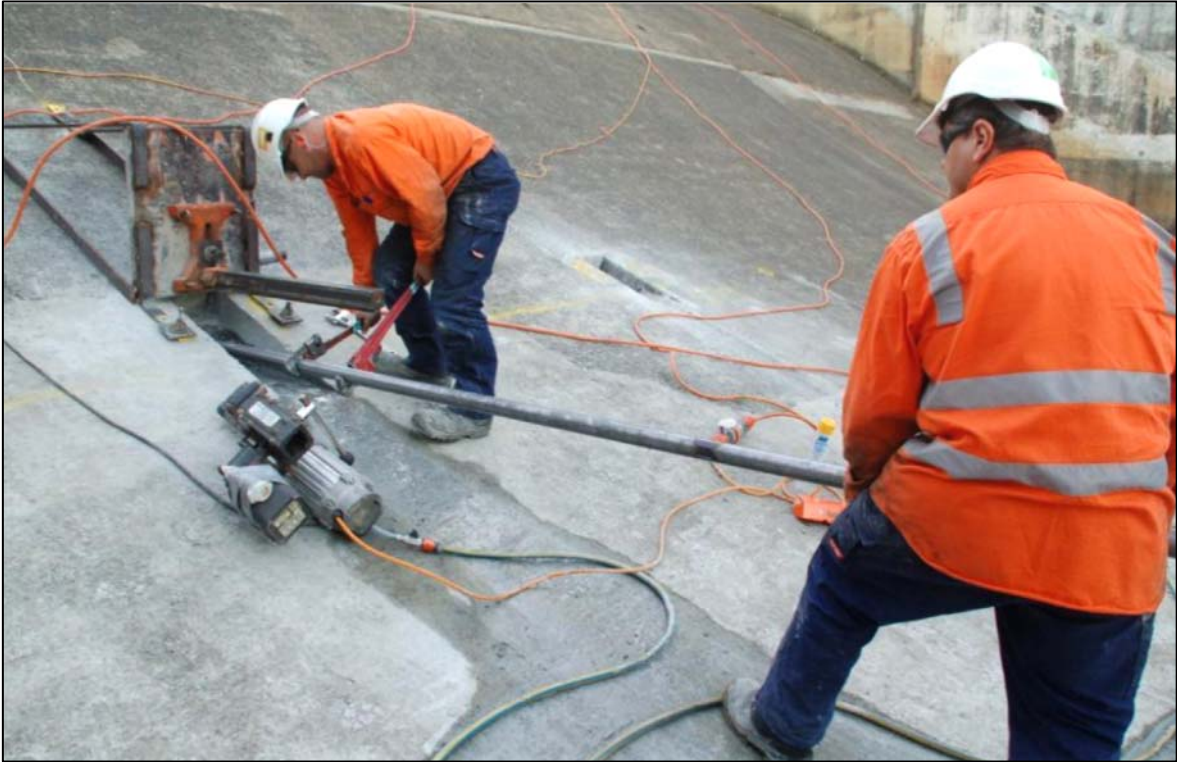
Each of the wire feed holes were drilled using continuous barrells. An accuracy of +/- 50mm was maintained in all drilled holes.
