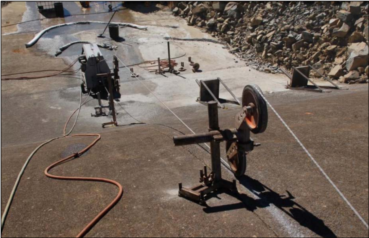
Tension is taken up and cutting begins all excess wire is taken up within the wire saw storage unit as the wire is continuously pulled through the concrete.
