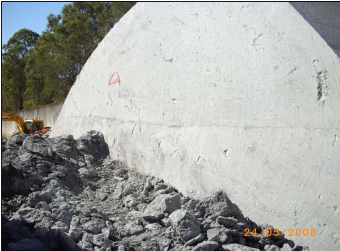
In all 240m 3 of concrete was removed each cut face was 14.5m long x 5m high approx. Allowing for the ogee shape a total of 48m 2 was cut on each face.
