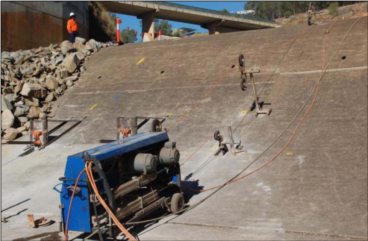
Wire saw was set-up and wire fed through the cored hole and back over top off ogee.
